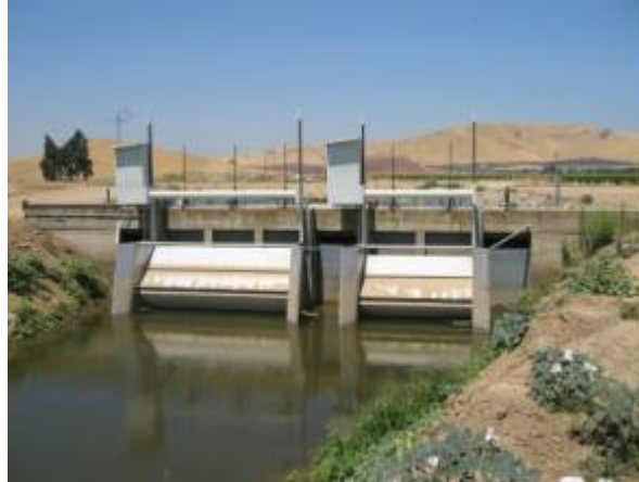
Figure 1. Before (top) and after (bottom) photos showing new Langemann gates at TID's entrance to the main canal at Rocky Ford. The Langemann gates are used for upstream water level control.
