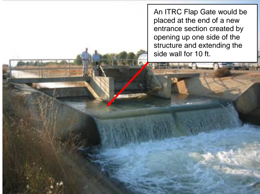
Figure 15. Downstream side of the Main Canal check structure showing where the ITRC Flap Gate is to be installed
