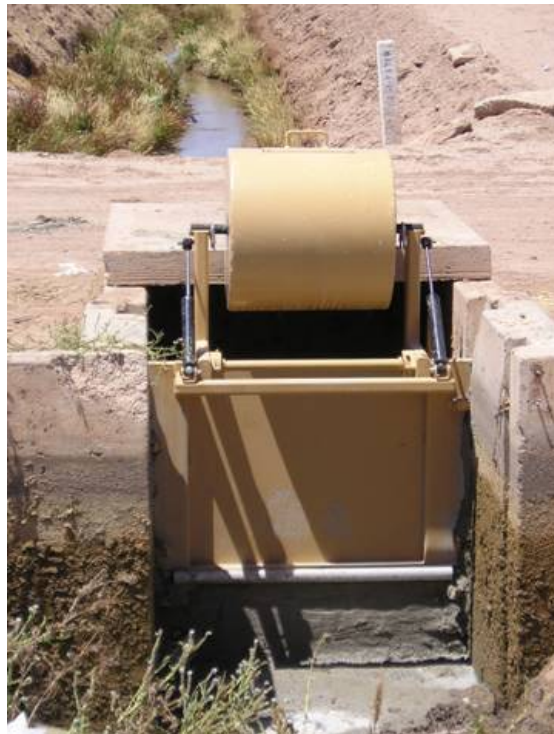
Figure 9. Example ITRC Flap Gate (Imperial Irrigation District). View from upstream.
