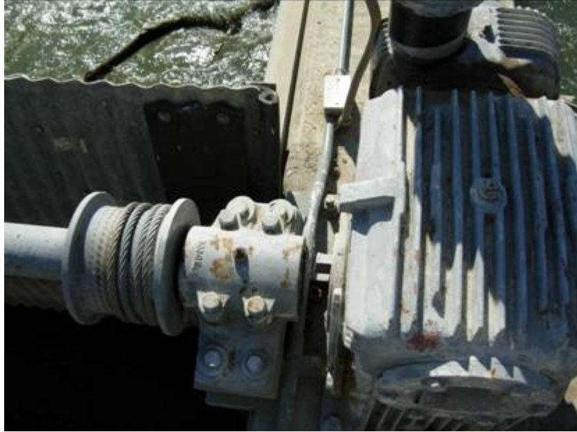
Figure 4. Short clearance at the end of the gate shaft for mounting an encoder to measure gate position (Willows Check)
