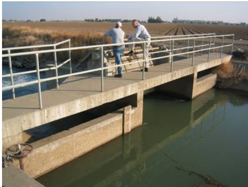
Figure 13. Main Canal check structure in the lower portion of the district (east of I-5)
