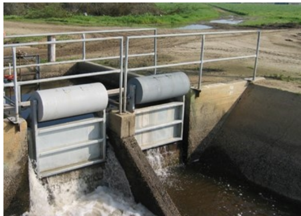
Figure 1. Galvanized “standard” flap gates without seals showing with some leakage at Chowchilla Water District, CA. It appears the gate on the left is operating and not fully closed, whereas the gate on the right seems to be fully closed.
