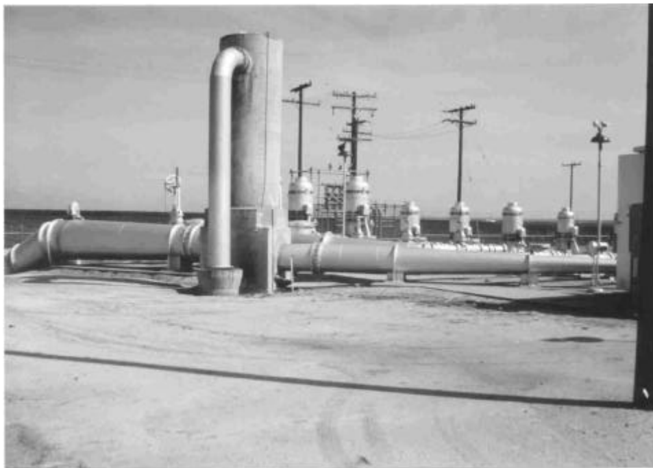
Figure I.6. Overflow stand at Station d12 to which the VFD was attached. The VFD maintains a constant water level in the stand, below the overflow pipe seen on the right hand side.
