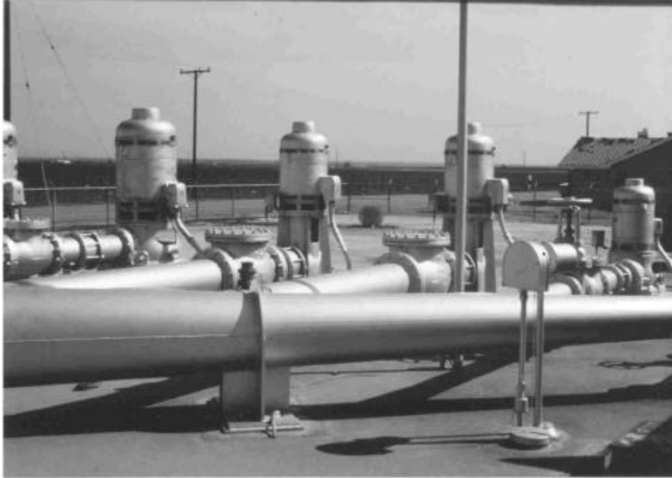
Figure I.1. Station D12. Pumps for the detailed study.
