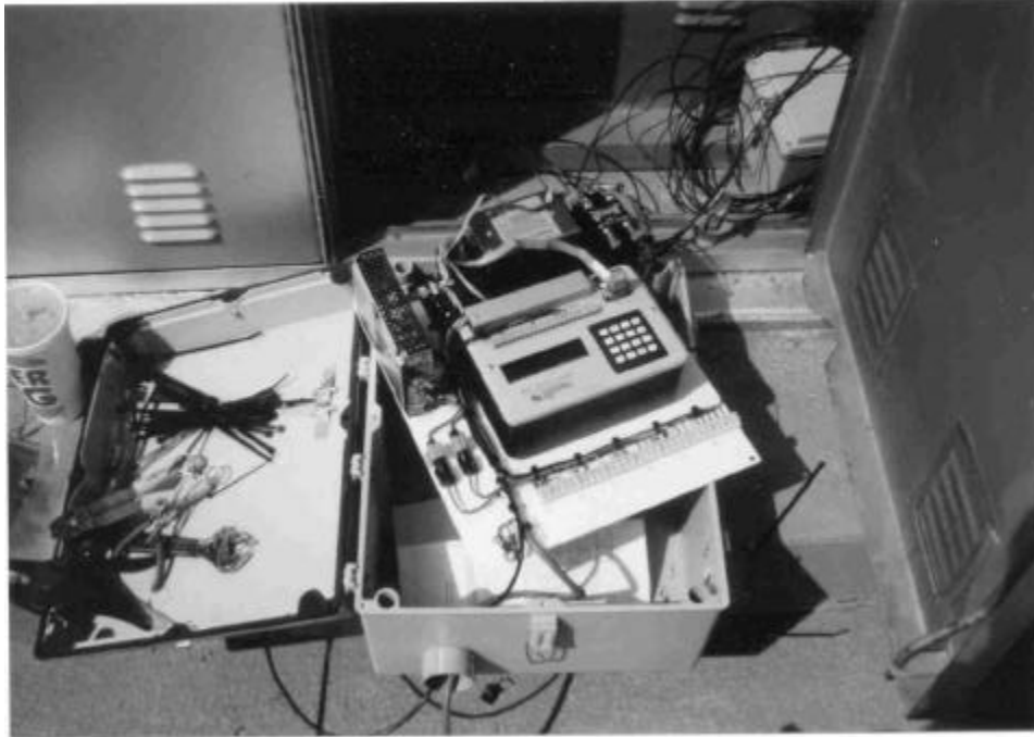
Figure I.3. Datalogger provided by SCE for data acquisition at Station D12.
