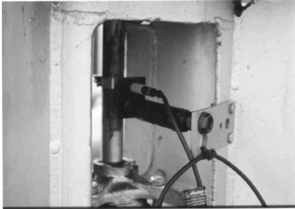
Figure I.5. Shaft RPM measurement device for the VFD pump at Station D12.
