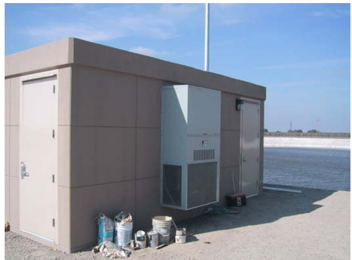
A new air conditioned enclosure for a VFD application at South San Joaquin ID.
